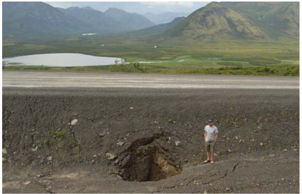
Fig. 3. A recurring sinkhole in the Dempster Highway embankment due to ground water flow at YT km 82 (2017).
