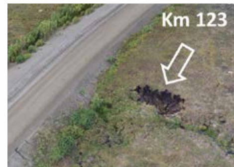
Fig. 18. Sinkhole forming due to thermal erosion at km 123, Dempster Highway.
